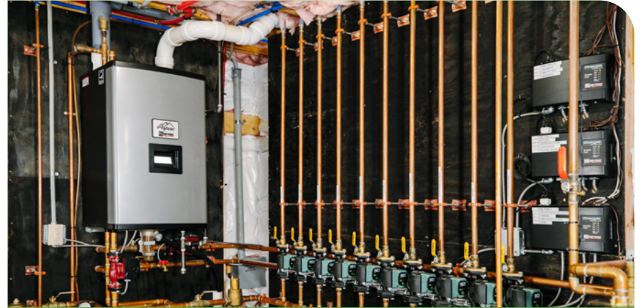
Long's heating system includes a condensing boiler, 10 hydronic zones, and two heat pumps for use in the shoulder seasons. A 70-gallon indirect water tank provides plenty of hot water for the multi-head shower in the primary bedroom suite.
