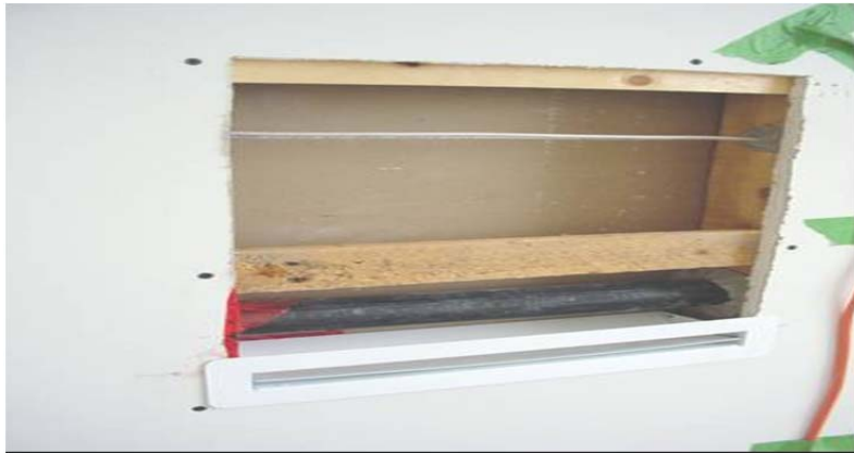
Figure 10: Photograph of Bedroom 2 Stud Space Openings around Electrical Wire
