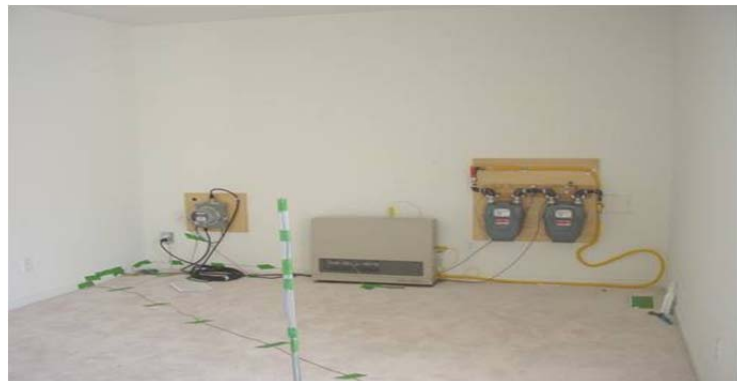
Figure 5: Photograph of Second Floor DV Unit in Master Bedroom against East Facing Exterior Wall
