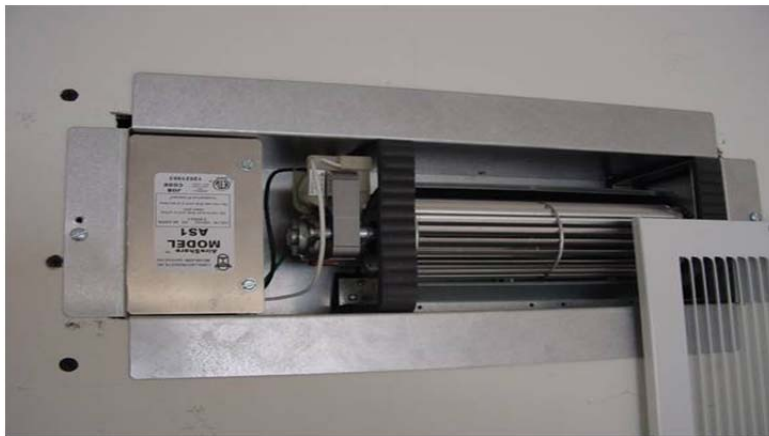
Figure 11: Picture Showing Air Share Grille Partially Removed
