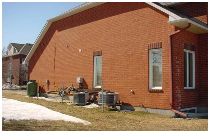
Figure 14: Photograph of Experiment House Exterior showing Propane Tank and Gas Tubing
