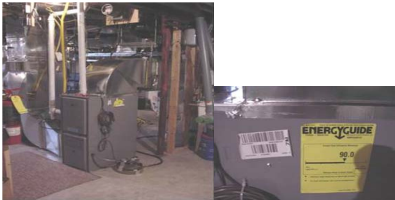
Figure 12: Photographs of Propane Furnace in Basement Connected to Existing Ductwork
