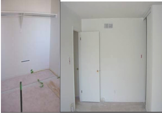
Figure 7: Photographs Showing Location of Air Share Intake Unit in Master Bedroom and Stud cavity in Bedroom 4
