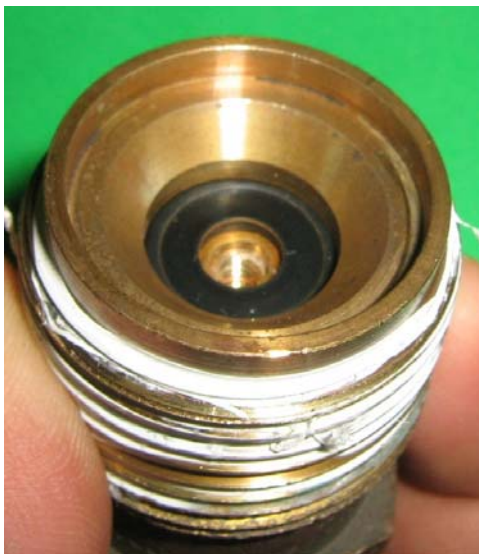
Figure C-42 - PRV 281 Gasket as Installed
