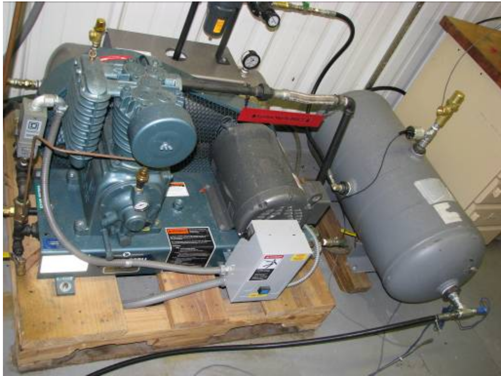
Figure 20. 500 psig storage tank and 300 psig compressor.
