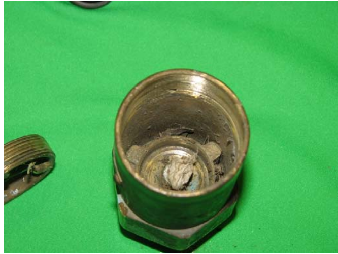
Figure C-20 - Debris inside PRV 80 After Spring Removal
