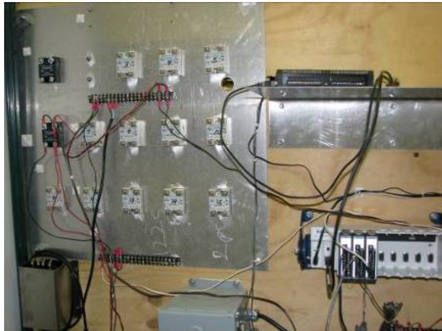
Figure 19. PRV test stand — electronics.
