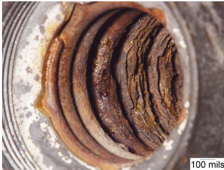
Figure A-2. Higher Magnification View of the Corrosion of the Coils in Spring in PRV 62
