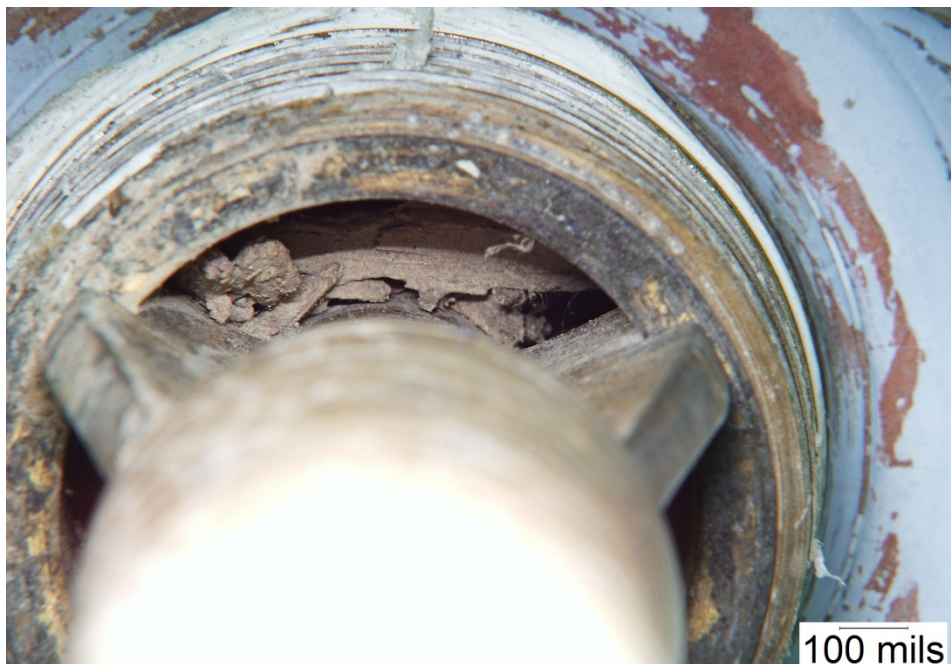
Figure A-30. Debris in the Valve Body Below the Sealing Surface
