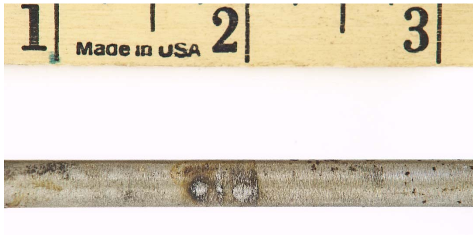
Figure A-23. Higher Magnification View of Some of the Corrosion on the Valve Stem from PRV 350
