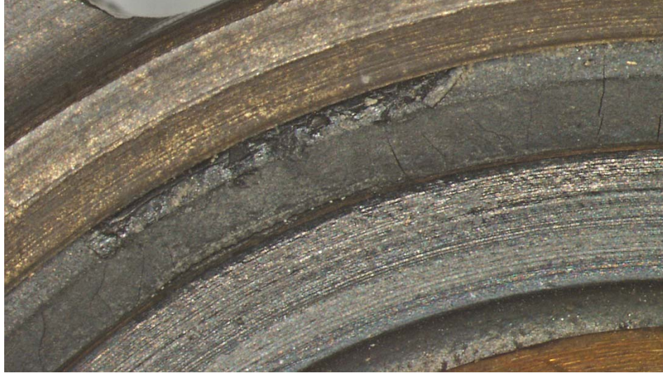
Figure A-37. Radial Cracks and Material Missing from the Outer Circumference of the Gasket from PRV 279
