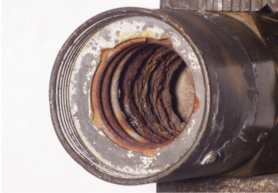
Figure A-1. Severe Corrosion of the Spring in PRV 62
