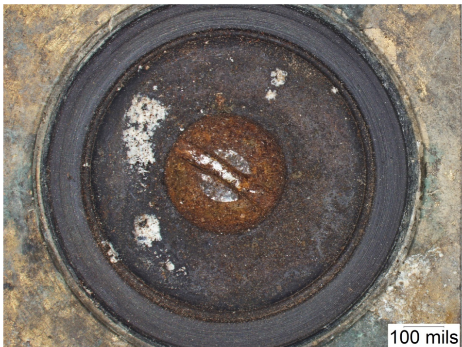
Figure A-5. Gasket Surface and Corroded Screw from PRV 62
