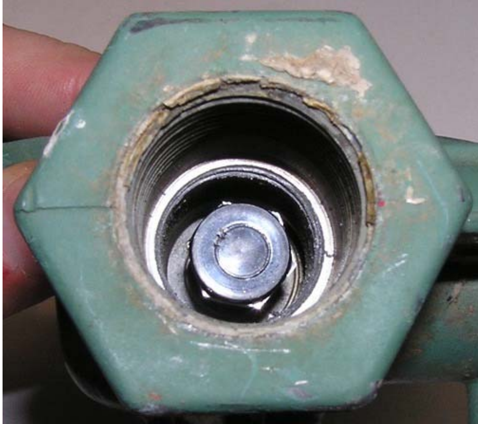
Figure 6: Damage to Inlet Seat Disc of Regulator #42
