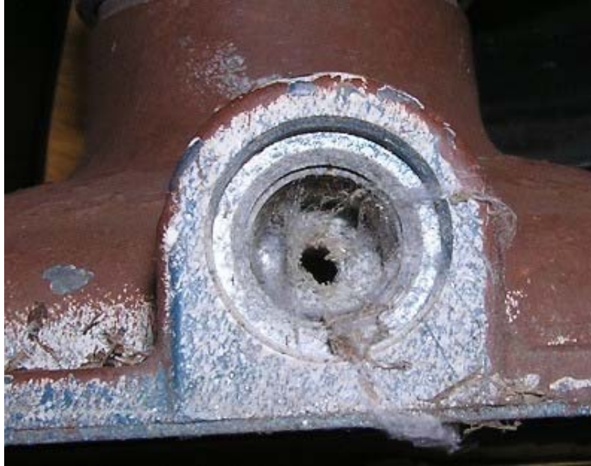
Figure 3: Regulator #711 Vent (After Cleaning)
