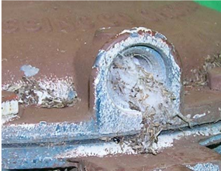
Figure 76. Regulator 711 — blocked pressure relief.
