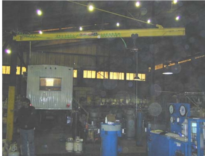
Figure A-5. Crane and chain hoist used to lift and lower propane tanks in and out of the water-filled jacket.
