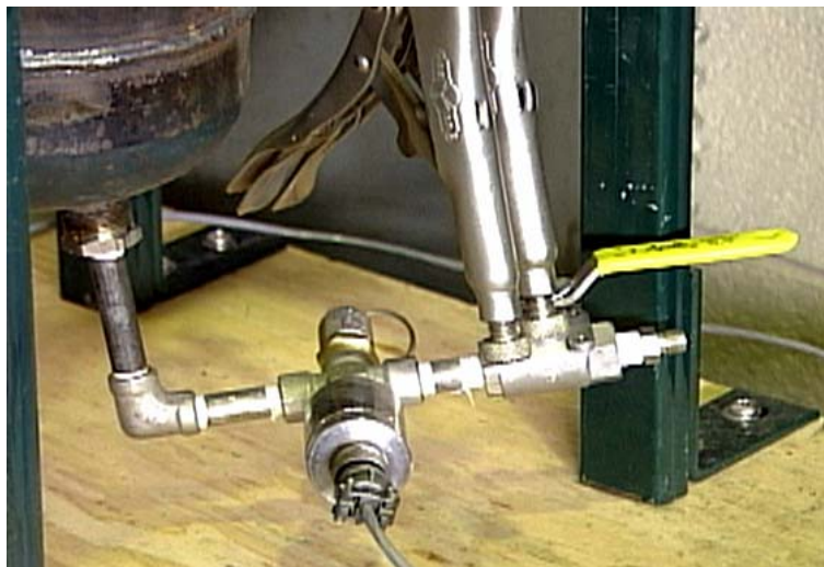
Figure A-14. Pressure transducer, manual valve and safety relief valve at the base of the test cylinder.
