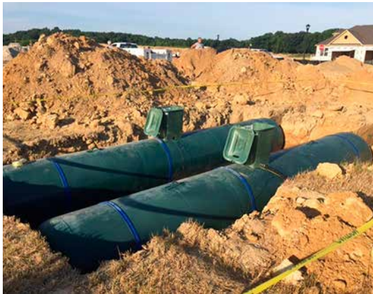
Each home at Bay Bridge Cove has an individually metered propane connection, with lines running to centralized propane storage tanks buried in common space. Homeowners are billed for propane by usage, just as they would be for natural gas service.
