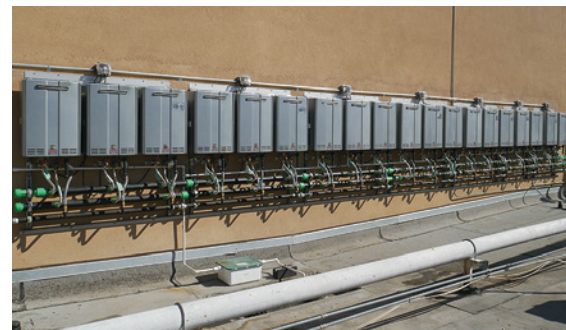
As the Pala Casino Spa and Resort grows for the future, tankless water heaters provide the uptime and reliability every facility manager craves.
