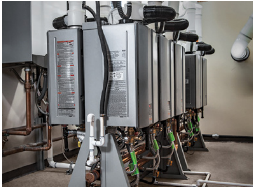
Tankless water heater arrays can be free-standing or wall-mounted and are available with common venting systems.
