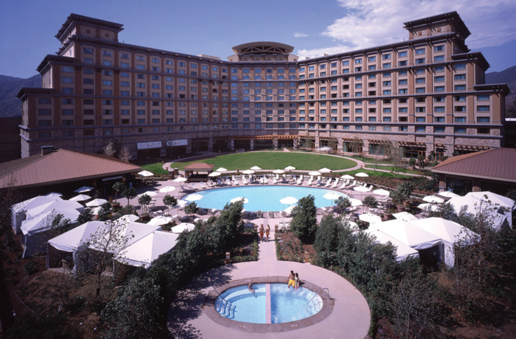
A propane tankless array serves all of the casino's potable hot-water needs, from the dishwashers to the restrooms.
