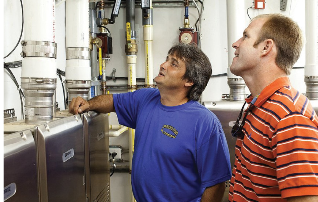
Contractor Anthony Crouch, owner of Crouch & Sons Plumbing in Florence, Alabama, examines the Residence Inn by Marriott's tankless water heater array with distributor Jason Veal of the Tallman Company. Photo credit: Randy Crow
