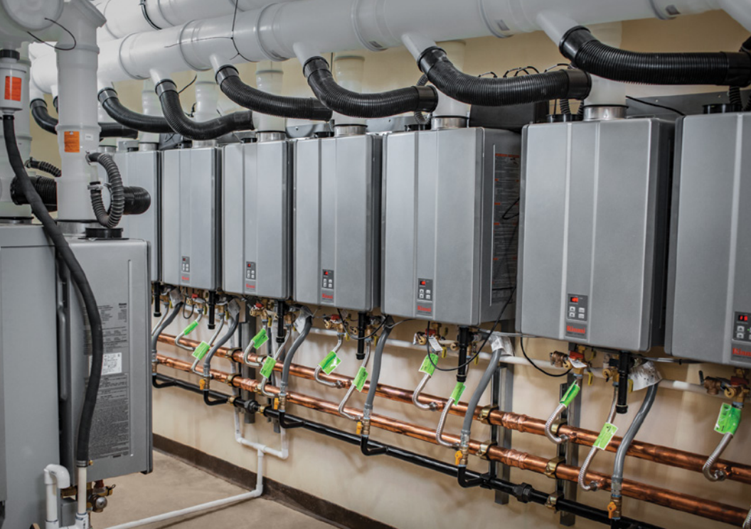
Using more-efficient tankless water heaters, Ruby's Inn is projected to save $6,000 a month in propane costs.
